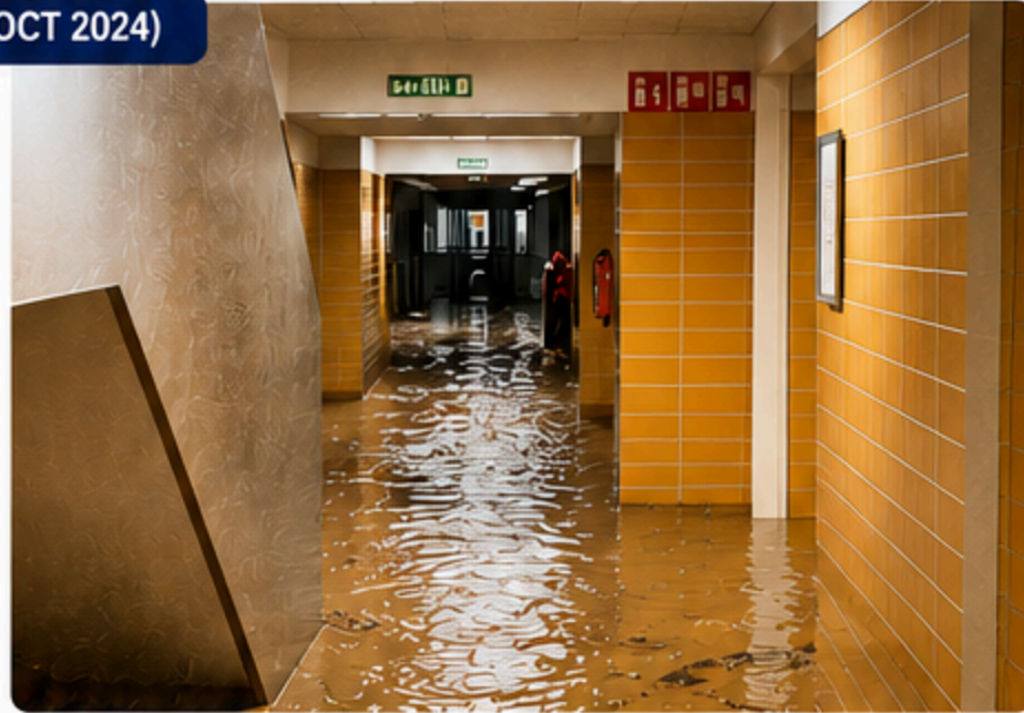
Primary care center affected during the Valencia DANA (2024).
