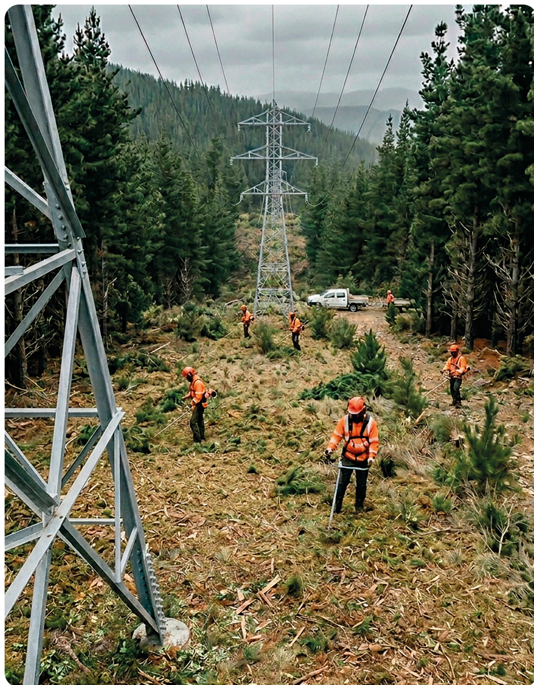
Field operations under live power lines — PPE visible
